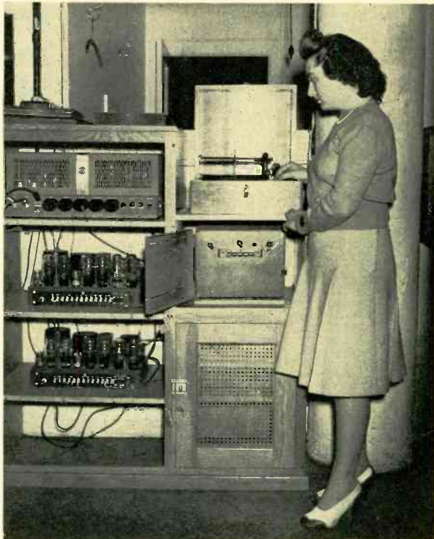
Typical public address unit is installed next to the works manager's office. This shows a four-network panel in the center compartment, and the attachment for playing records (bought outright or rented from the dealer) is directly over.
